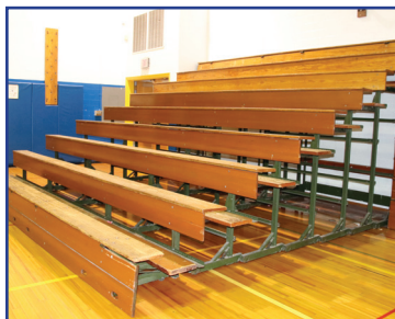
Bleacher Replacement Replacement of the original bleachers at Spry MS will provide safety features such as railings.
